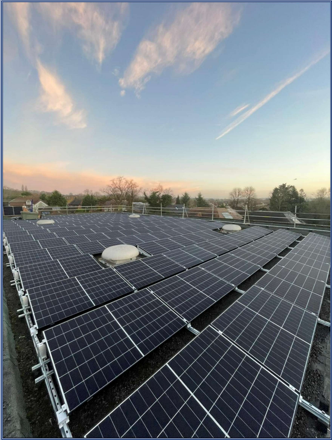
Sunrise over our new solar installation installed in January 2026
